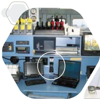
Communications centre on the bridge, FleetBroadband handset (circled).
